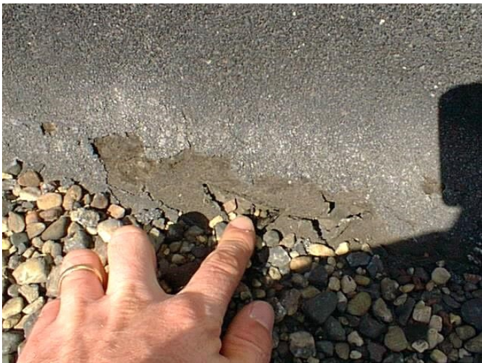
F-102 Field Membrane - puncture/Hole/tear # 3 All holes in the membrane are considered high severity due to their high leak potential.
