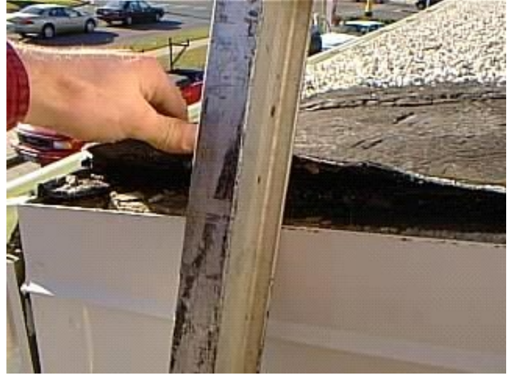
ME-100 Metal Edge - deteriorated membrane # 2 The flashing membrane is deteriorated and should be replaced to avoid further degradation.
