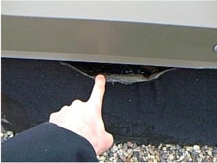
BF-110 Base Flashing - open lap # 1 Seam in flashing is open through entire width, allowing water to penetrate the flashing.
