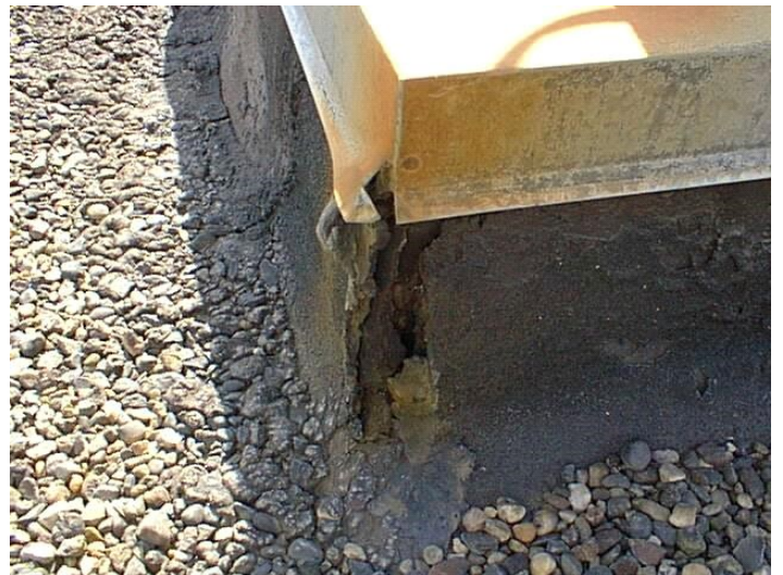
P-100 Penetration - deteriorated membrane # 4 The flashing membrane is deteriorated and should be replaced to avoid further degradation.
